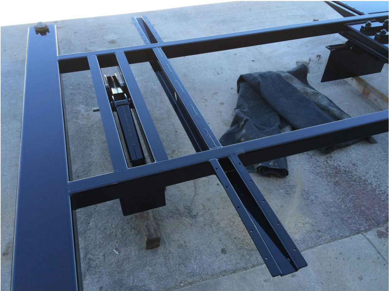
Building of the subframe begins and is delivered to Crump Truck in Oct. 2015
