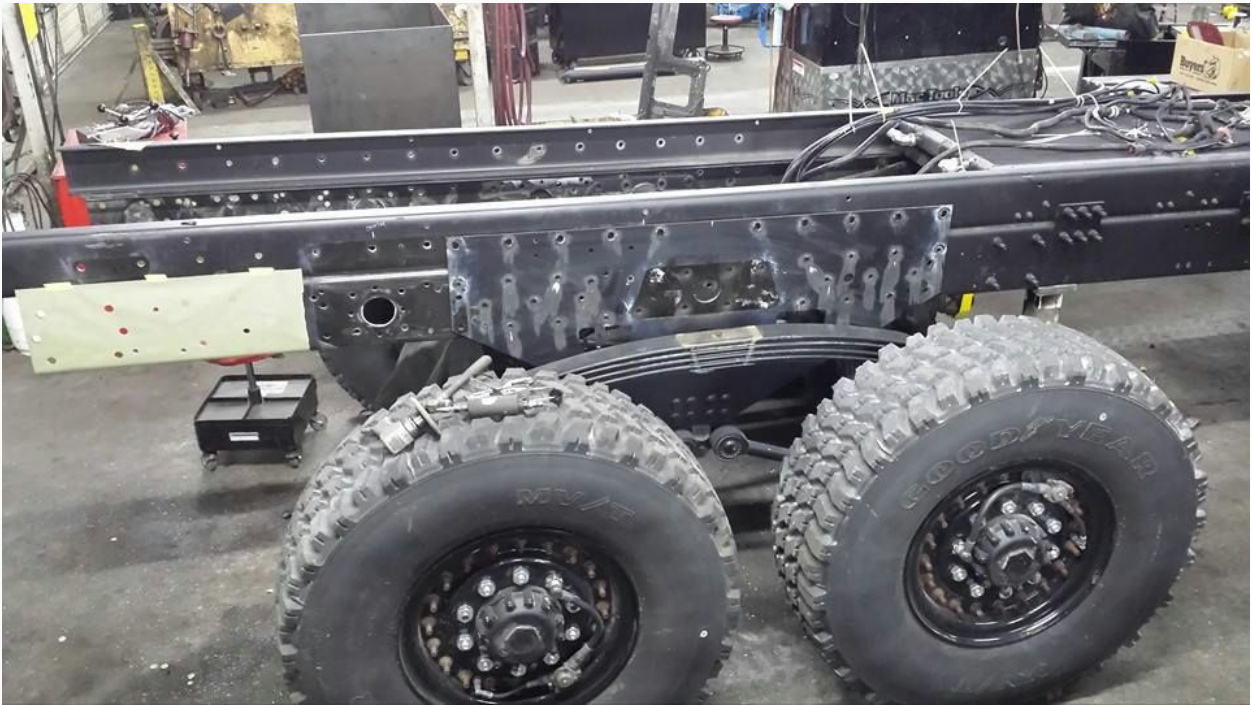
Cutting the rear suspension loose and drilling holes for a longer wheel base.
